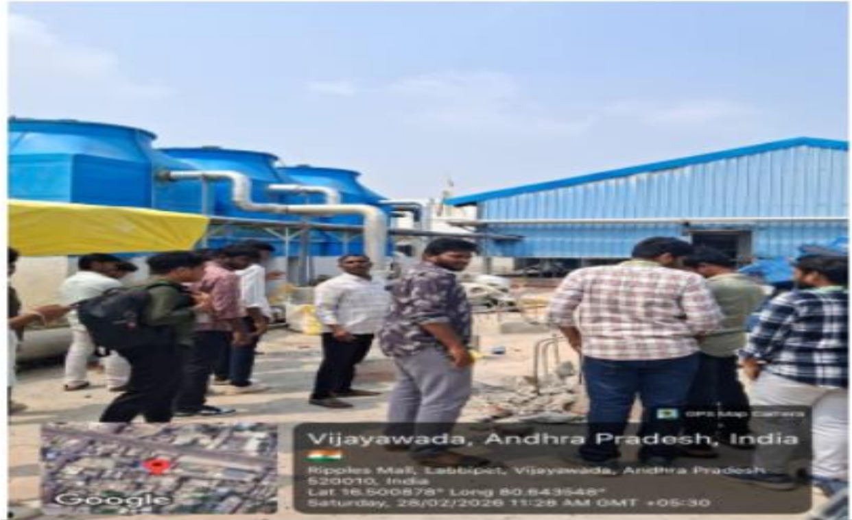
ISHRAE students in front of Air/water cooled chiller plant
